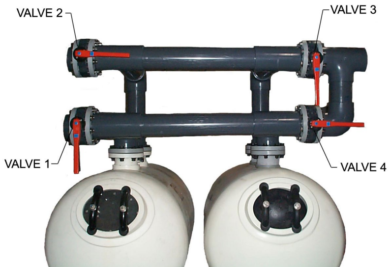
Dual Tank System Piping at Right (Filter Mode)
