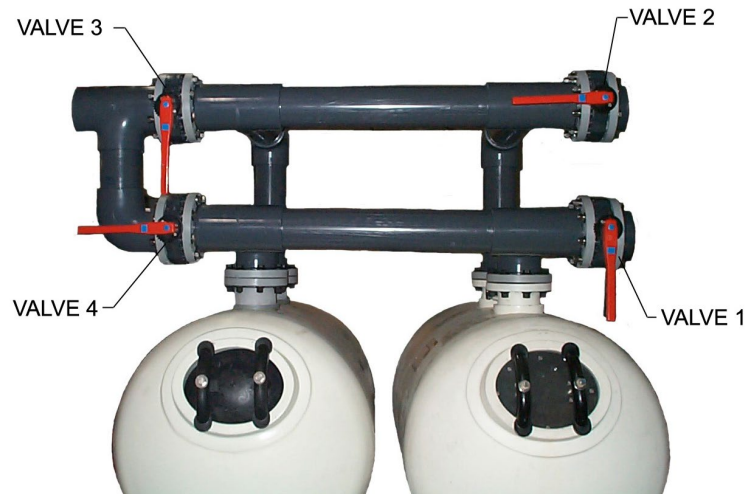
Dual Tank System Piping at Left (Filter Mode)
