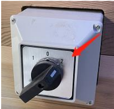
Power to Infrared heaters
