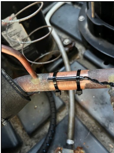
Figure 14- Sensor on Suction Line
