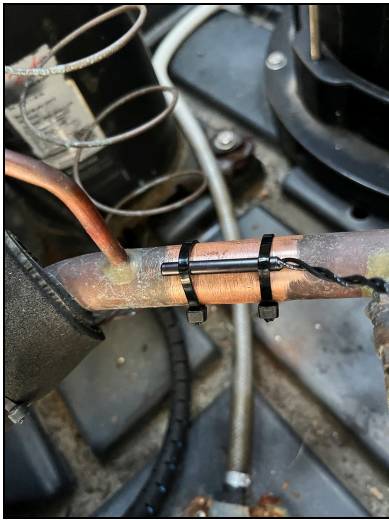
Figure 13- Sensor on Suction Line
